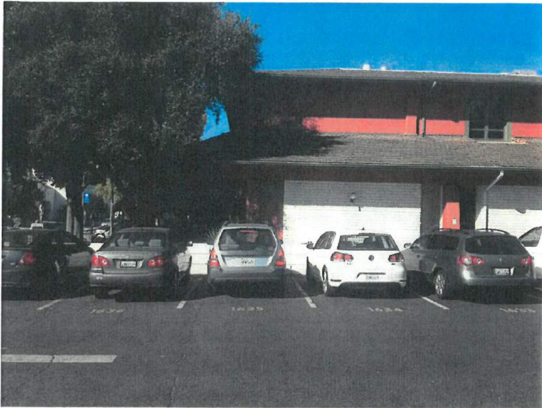
Photo 2. Southeast Corner of East Wall First floor CMU walls (white) are between concrete columns and a concrete beam above (red). The second story is set back 15'-6" from this wall and has concrete perimeter walls (red).
